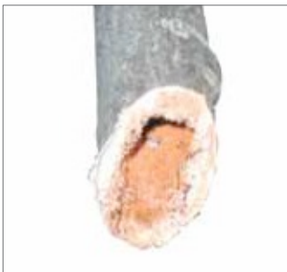
Corrosion build-up in metal pipes
