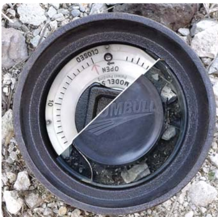
DEBRIS SHIELD keeps dirt off of Position Indicator, as the composite image shows above. Note how white color illuminates inside valve box!
